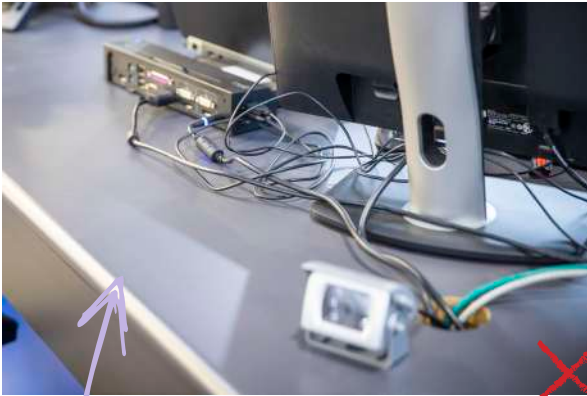
Cords need to be kept tidy at all times and cable ties are to be used where needed
